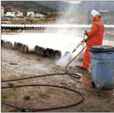
Here is an example of water blasting pipes using VpCI®-611 to protect the uncoated surfaces.
